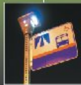
Solar Transit Lighting
