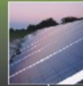
Industrial Solar Power Systems
